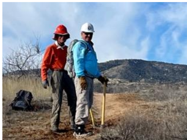
Ray Peale and Steve Aiken working on drainages along the Arizona Trail. Photo by Elisabeth Wheeler
